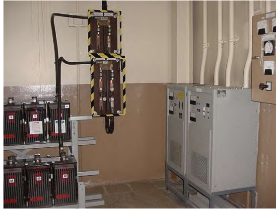
Fig. 18. Substation Auxiliary DC Equipment
