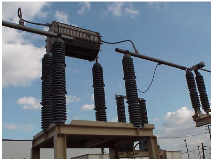
Fig. 13. Free Standing 138 kV 2000 A Wave Trap
