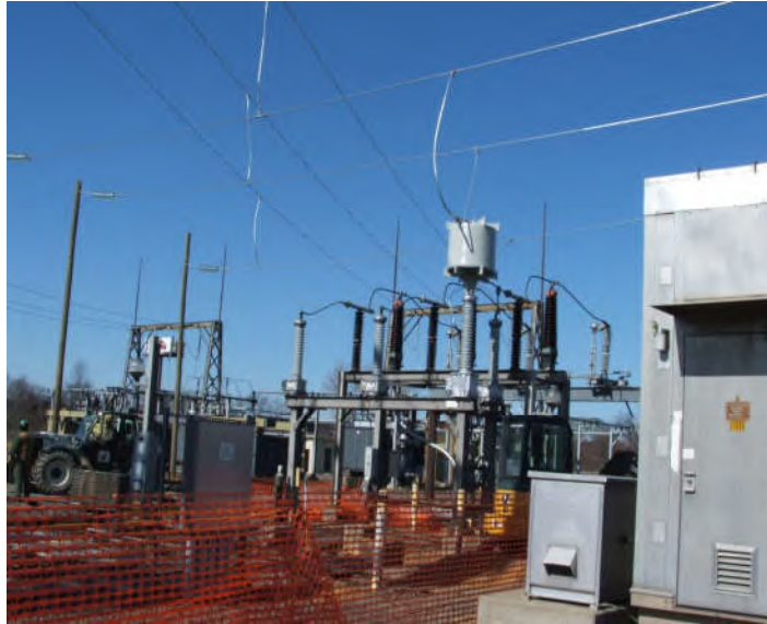
Fig. 12. 138 kV CCVT with 3000 A Wave Trap
