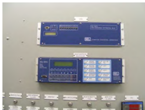
Fig. 2. Microprocessor Relays Installed on the Panel
