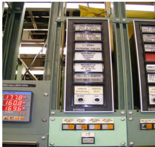
Fig. 19. 6- Window Substation Annunciator
